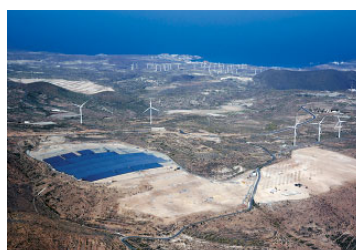
Bird's-eye view of the solar power generation plant in Tenerife (under construction)
