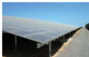
Solar Power-generating Facility in Spain
