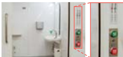
Wheelchair users also find these open/close switches easy to use
