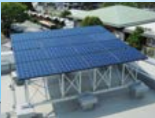
Rooftop solar power system
