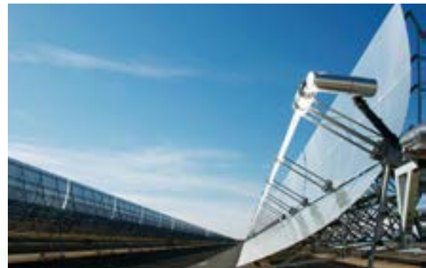
Solacor solar thermal power plant (Photo by Courtesy of Abengoa Solar)
