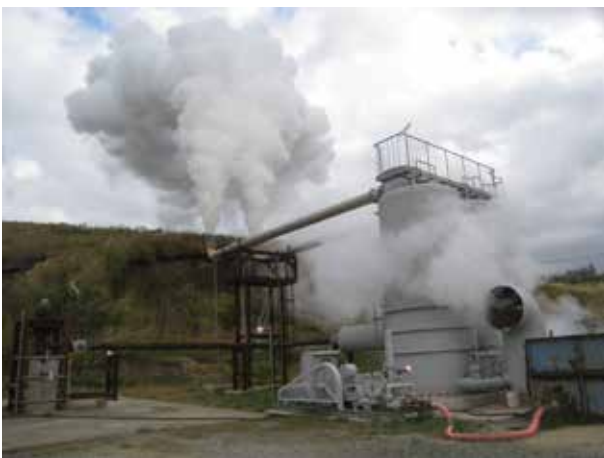
Steam output test (Source: Kyushu Electric Power Co., Inc., materials)
