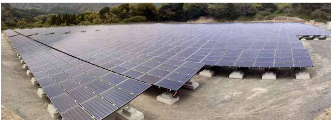
The solar power generation facility to be operated by the project
