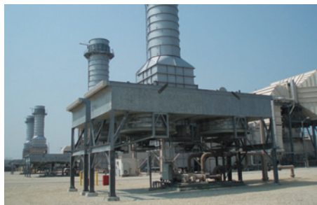
Elwood Energy power generation facility acquired by J-Power USA
